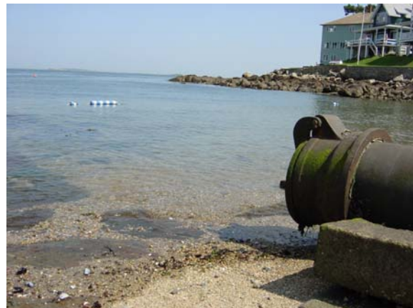
A stormwater outfall pipe at Juniper Beach in Salem, one of the many sites monitored within the Clean Beaches & Streams Program.
