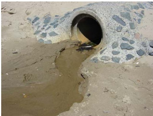
Dry weather drainage from the pipe at Brackenberry Beach, Beverly, taking the form of a small stream running across the beach.
